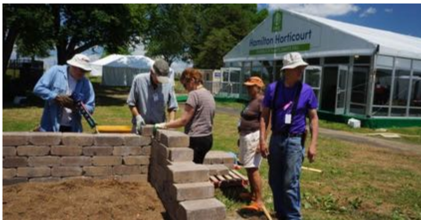
Installation crew at work (from left): Stuart Brooks, Michael Martin Mills, Maris Ogg, Linda Hartnett, Ron Rabideau
